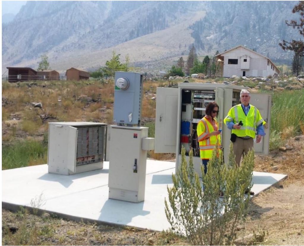
Viewing a remote terminal in Swall Meadows that provides phone and Internet service in area burned during Round Fire, February 2015
