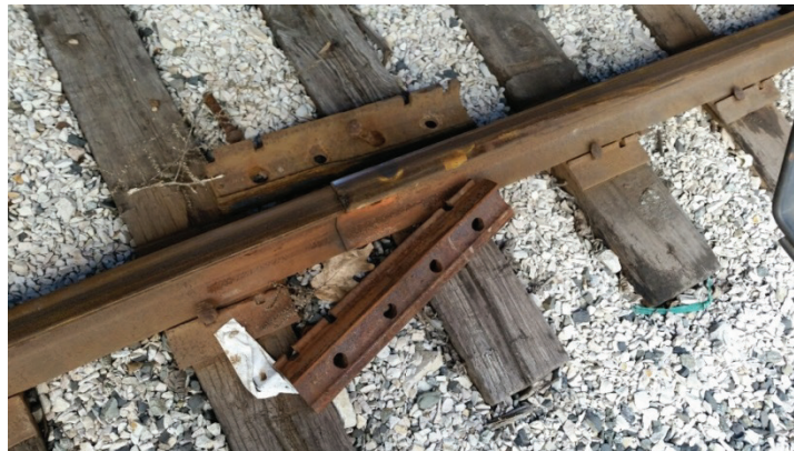
Close-up view of angle bars that were found lying on the ground.
