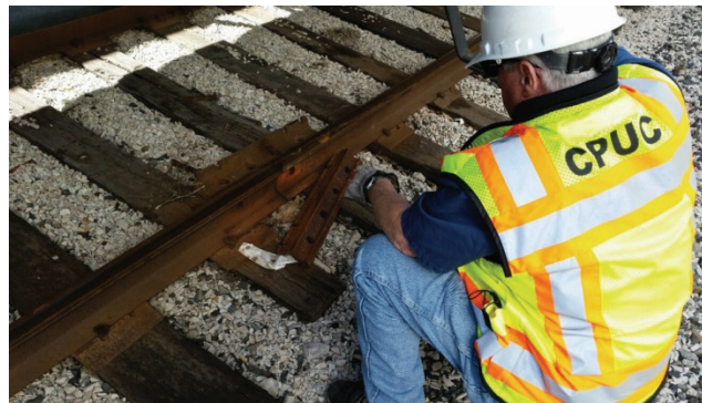
CPUC Rail Safety Inspector notes angle bars that are not bolted directly.
