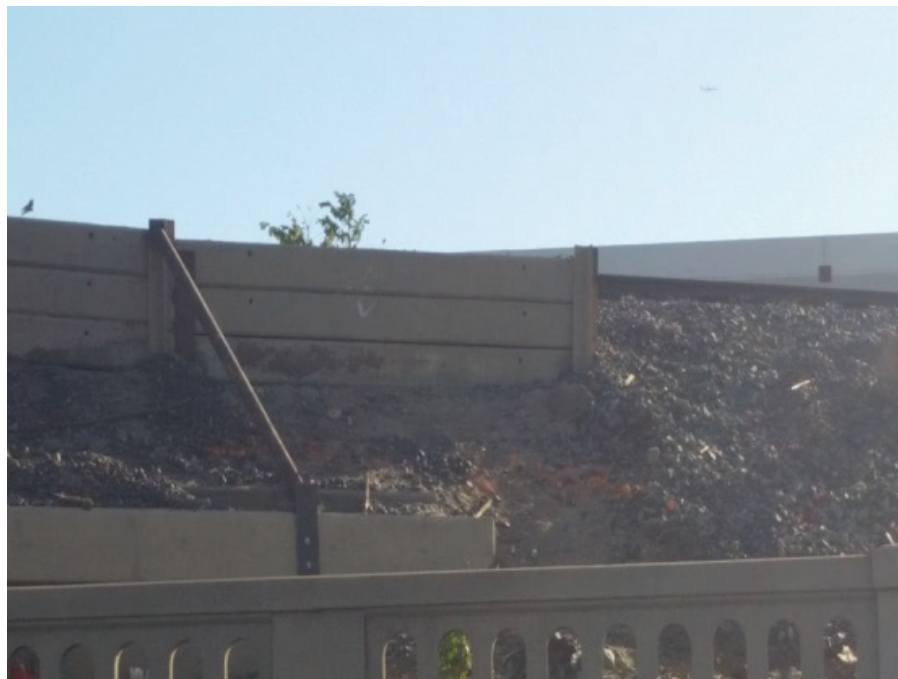
Top: "Before." Photo illustrates the concrete block from the retaining wall that could be dislodged in the event of an earthquake or adverse weather conditions. Bottom: "After" photo illustrating the repaired retaining wall.
