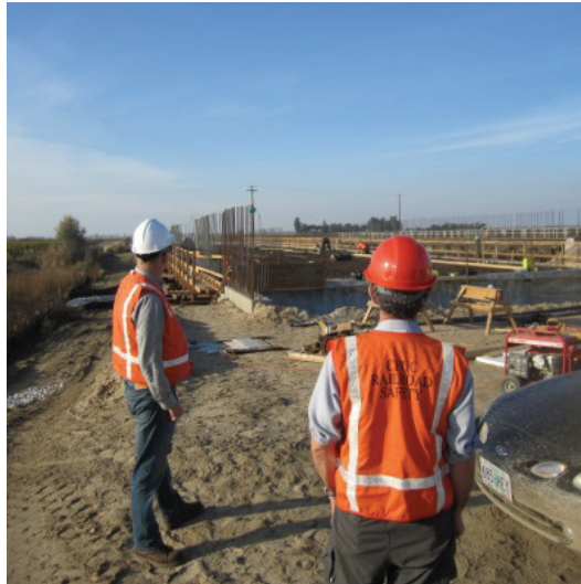
CPUC HSR staff observing construction of the Cottonwood Creek bridge near Madera, CA.
