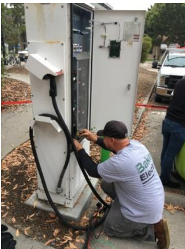
a) Connecting the CA-10 to the external load bank
