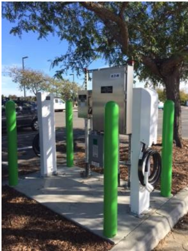
a) Nuvve PowerPorts at P703 Parking Lot
