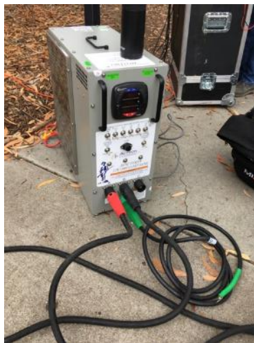
b) Load bank and wiring to data collector and CA-10
