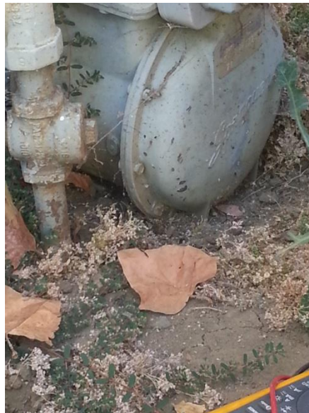
Photo 1. Buried meter at 23 Elm Street, Winters
