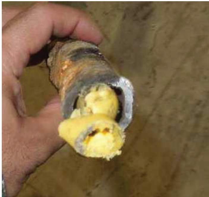
Figure 5: The service riser inserted with plastic.
