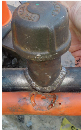
Figure 1. Damaged plastic service line insert and the tapping fitting welded onto the steel casing.
