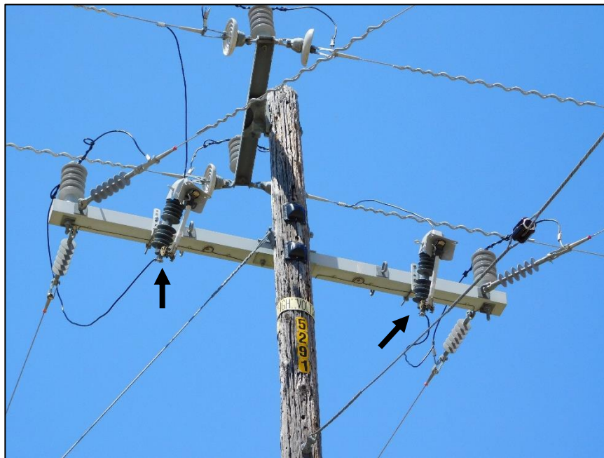
Figure 10: Old Pole/New Crossarms/Non-Exempt Fuses
