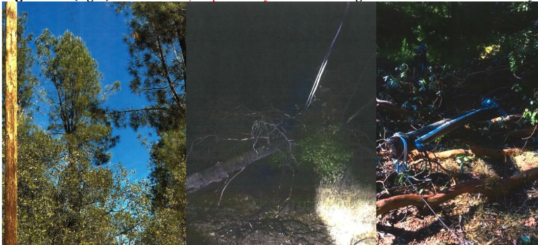
Figure 10: (right) In Yountville, Napa County Related Damage – Tree took down secondary pole
