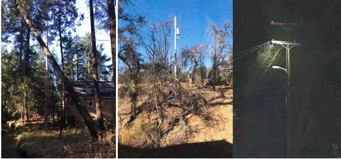
Figure 7: (right) In Clearlake, Lake County Veg Related Damage – Tree limbs fell on service wire, disconnecting it from pole
