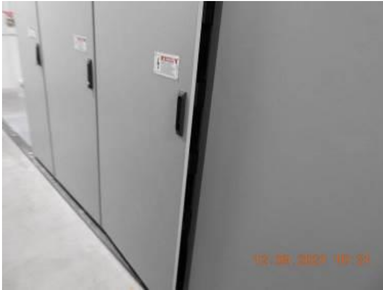
Broken handle preventing door from closing properly.
