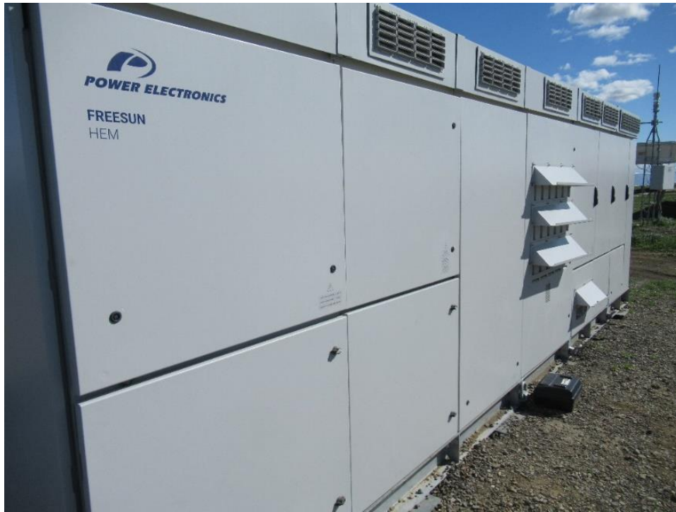
Figure 2: Missing signs/labels on one inverter
