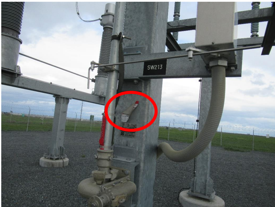
Figure 1: Peeling Arc Flash Label
