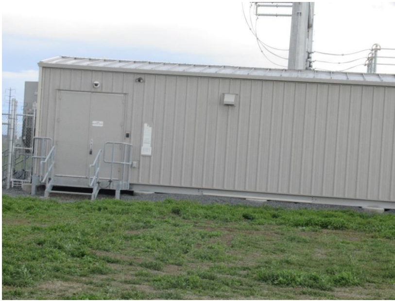
Figure 3: Missing NFPA sign (fire diamond) near entrance of control room
