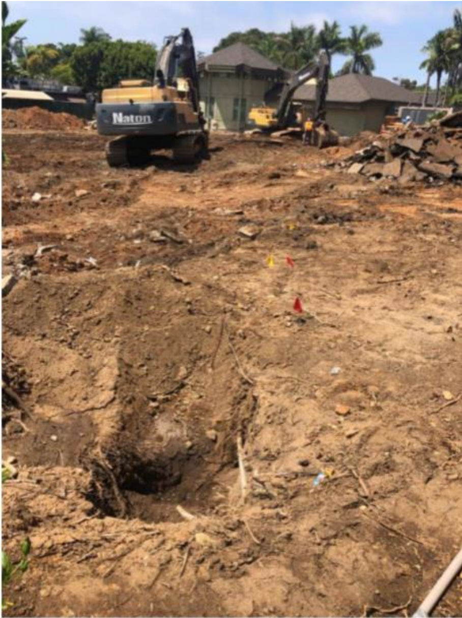
Image 8: Flags in area described on expired USA Ticket #A191060668 labeled Cable, Pipe and Leak.
