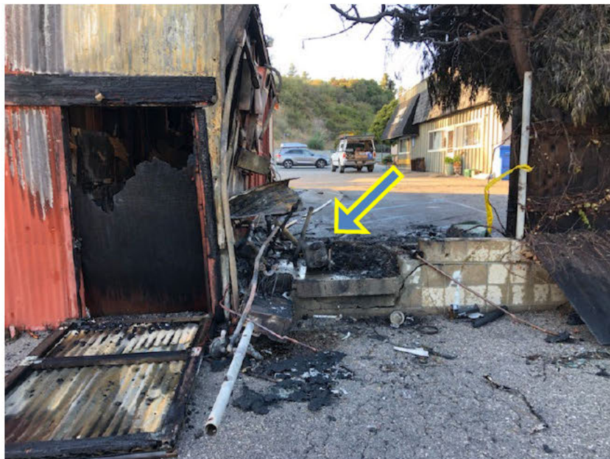
Looking from Museum Alley toward Main Street. Arrow to damaged MSA
