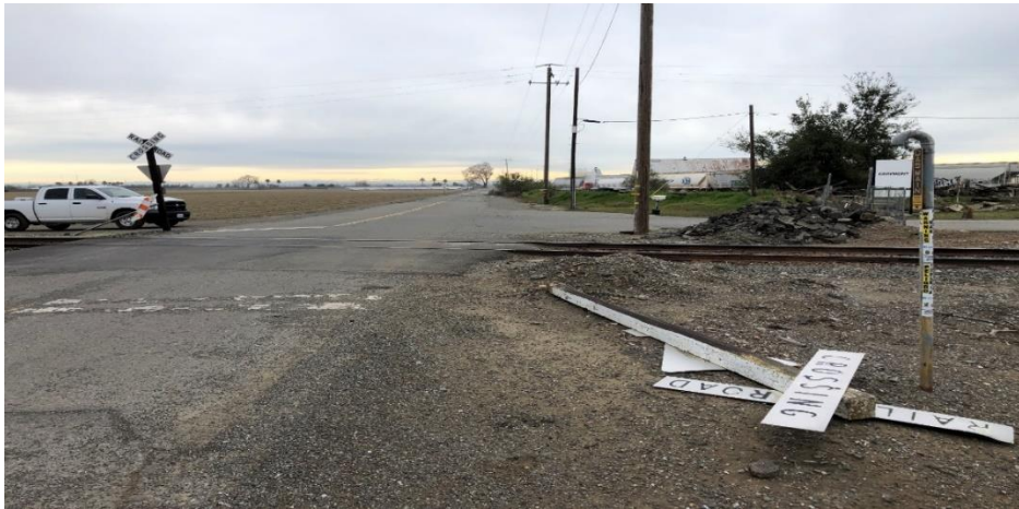
Before: Passive warning device, the crossbuck protecting the west side of the grade crossing at Best Ranch Rd (Co Rd18A) was knocked over and is no longer providing warning to pedestrians or vehicular traffic.
