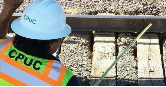
A CPUC inspector pointing at the broken rail
