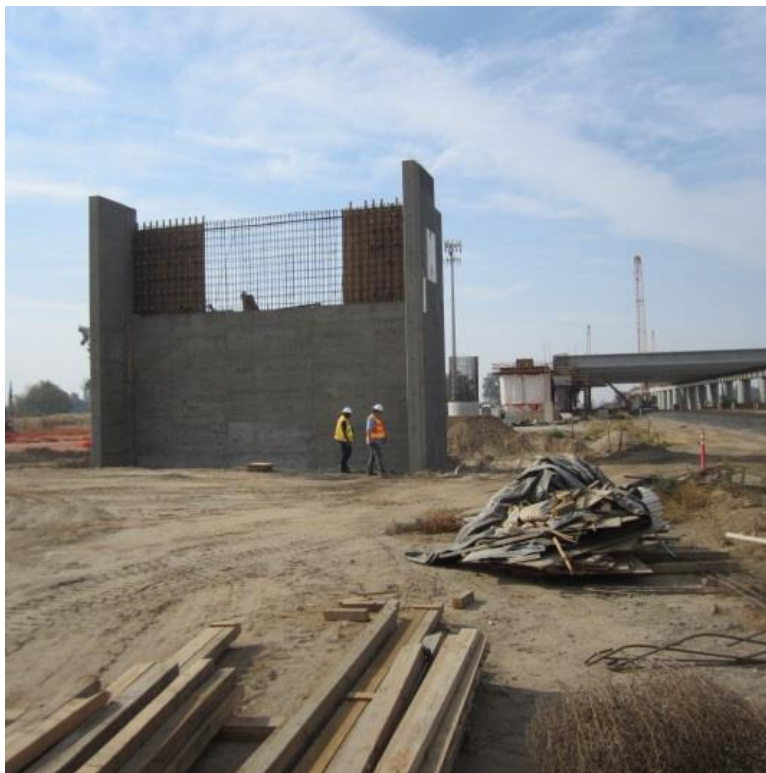
CPUC staff at the San Joaquin River Pergola and Viaduct construction site
