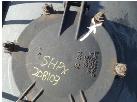
Example of loose bolt marked for tightening
