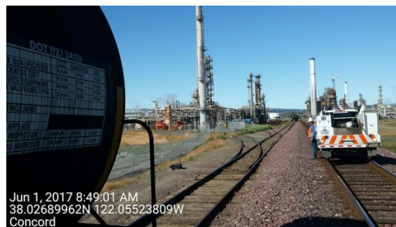
Another view of how close the defective rail was to the BNSF 70 mph main track, and its proximity to the Tesoro Refinery in Martinez
