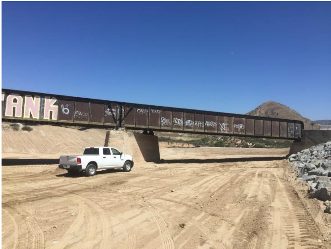
The same bridge after the BNSF Railway dredged out the silt to allow for more adequate water flow
