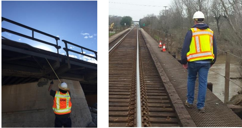
CPUC railroad safety bridge inspectors review bridge structure integrity and associated potential risks during field inspections
