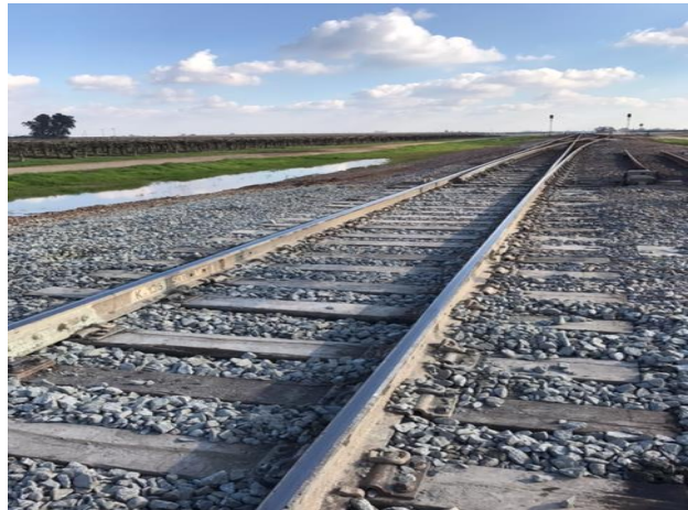
After: The ballast was replaced to provide greater stability to the track.
