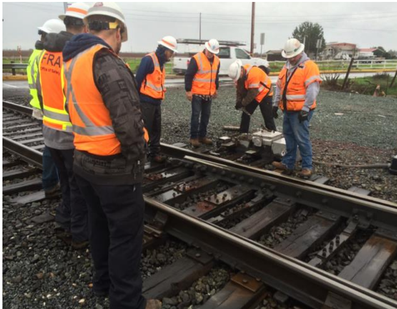
CPUC and FRA inspectors observing a BNSF signal maintainer adjusting a power switch machine
