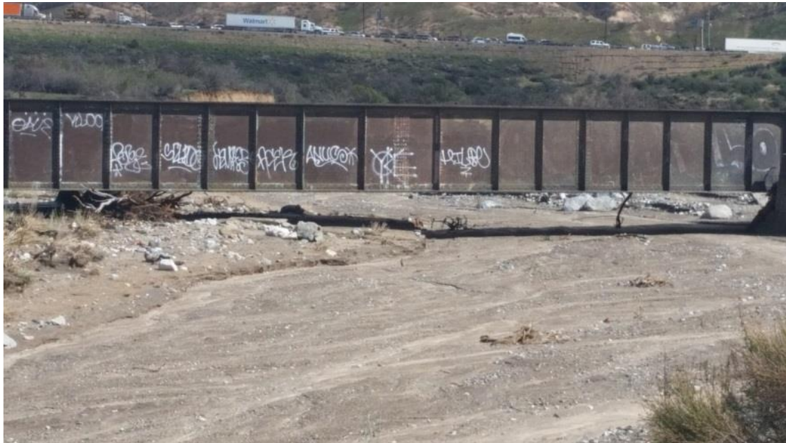
BNSF Railway Bridge at Cajon Creek, showing poor separation between the stream bed and the bottom of the bridge
