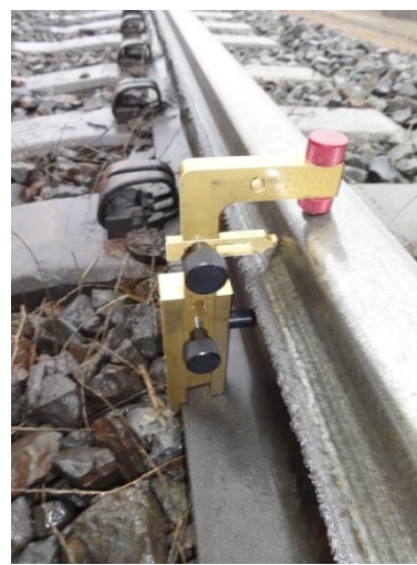
Rail head wear gage depicting 22/32" wear loss
