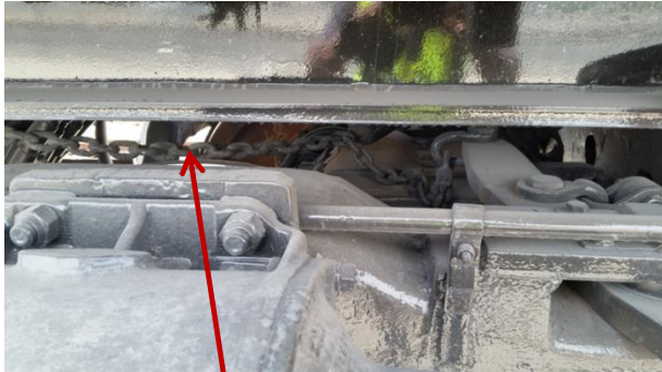
Before: The handbrake is not applied. Note the slack (dangling) in the chain, which indicates the hand brake is not applied
