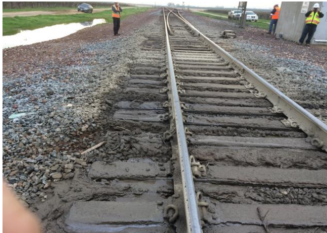
Before: The ballast does not provide adequate drainage because it is “fouled” or contaminated with dirt and mud. It cannot provide adequate support for the track and can cause misalignment of the power switch, which could cause a derailment.
