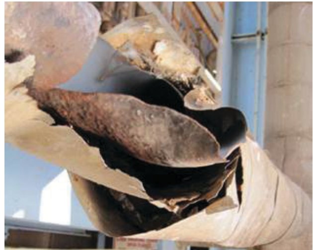
Pipe damage due to hidden corrosion
