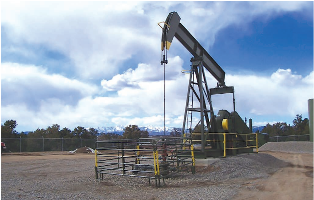
Pumpjack located on the Southern Ute Indian Reservation
