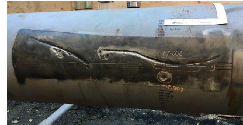
Defects found on Transmission Pipeline
