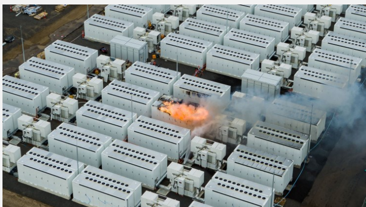
Figure 56: Victorian Big Battery Project event (July 2021).
