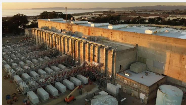
Figure 57: Moss 300/Dallas Energy Storage installation.
